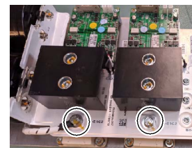
SC13 Busbar IGBT
