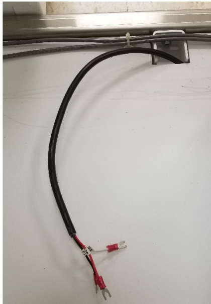
Figure 28: Foot Switch Cable Routing
