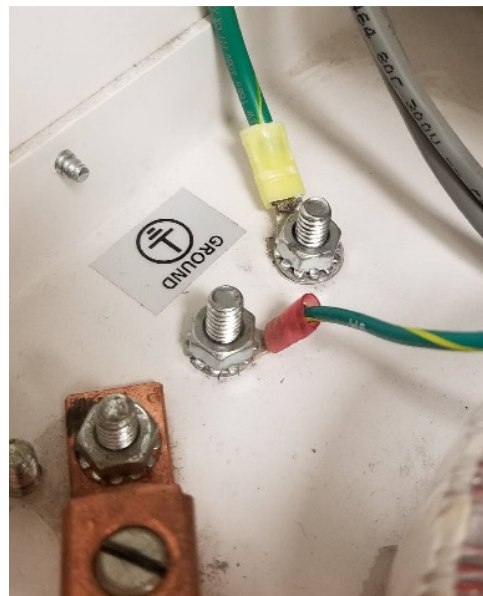
Figure 24: Earth connection in generator
