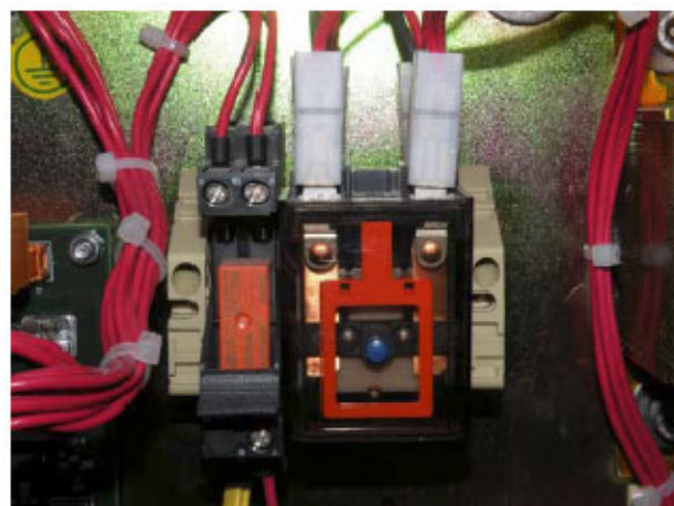
Connection after bypass
