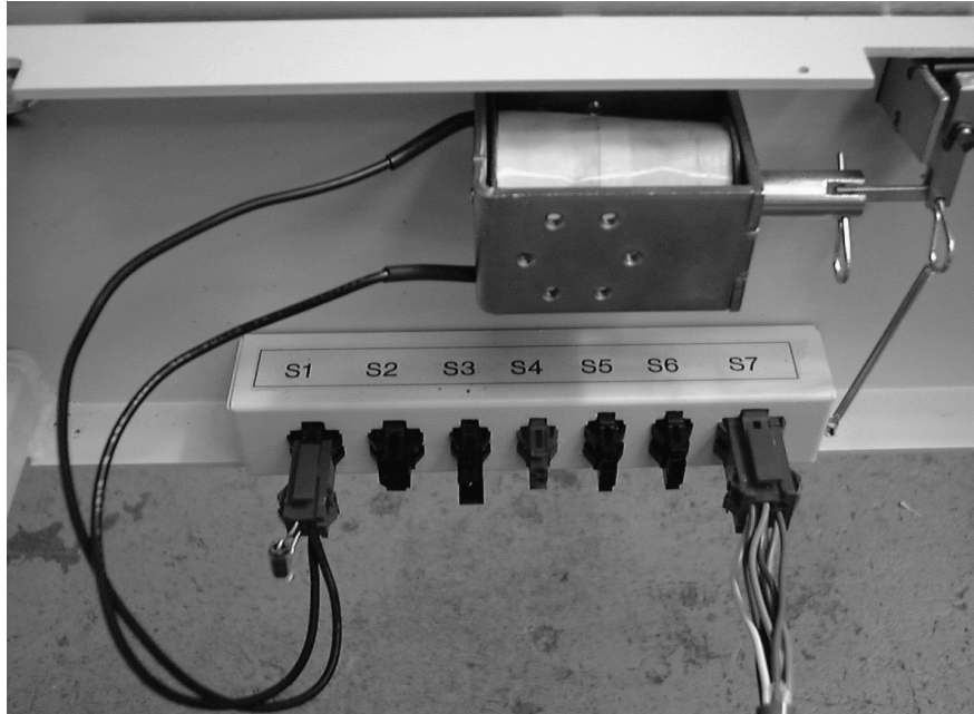
Figure 16: Table Interface Junction Box
